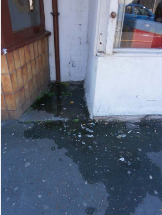
1) Overflowing drainage to front of premise
