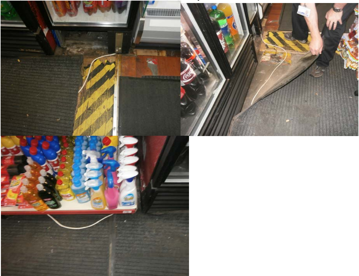
2) Cable run under carpets and across walkways.
